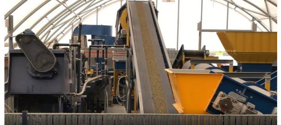
Figure 28 – Glass crushing machine, West Nowra
